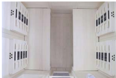
Overhead view Note vented inset heaters
